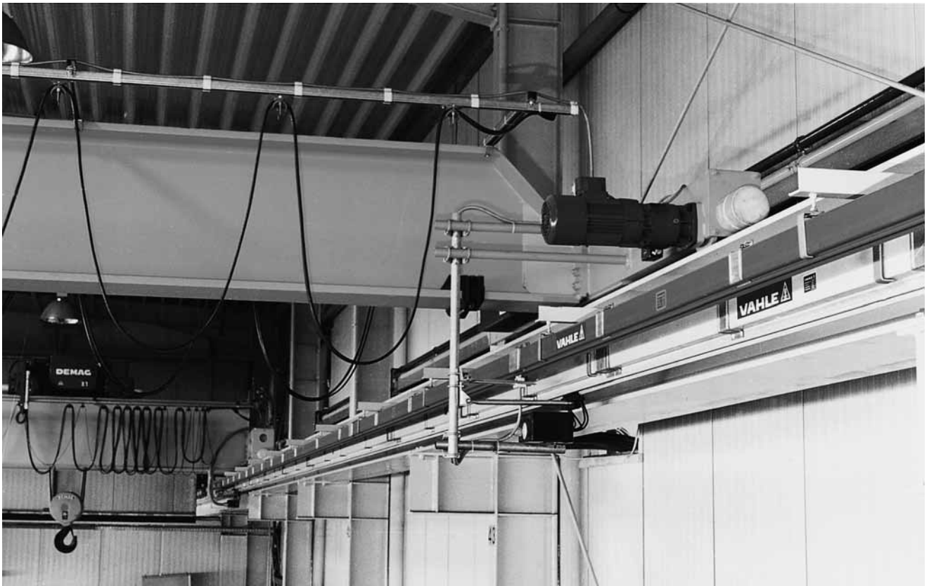
Power rail for the current supply of a hangar crane.
